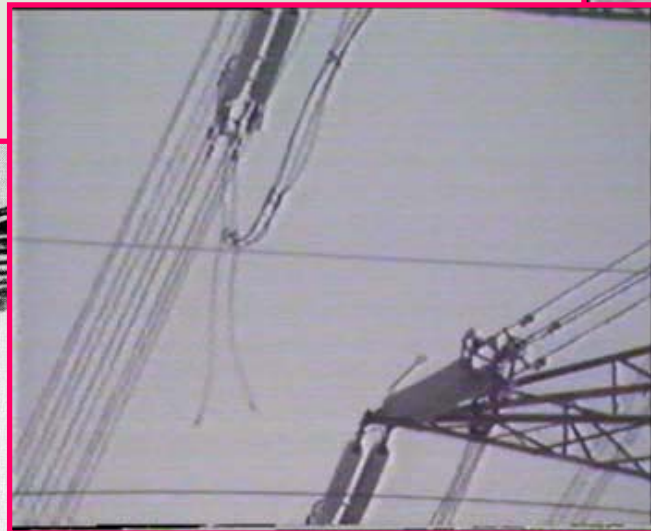
JUMPER LOOPS OF QUAD BUNDLE BROKEN DUE TO GALLOPING
