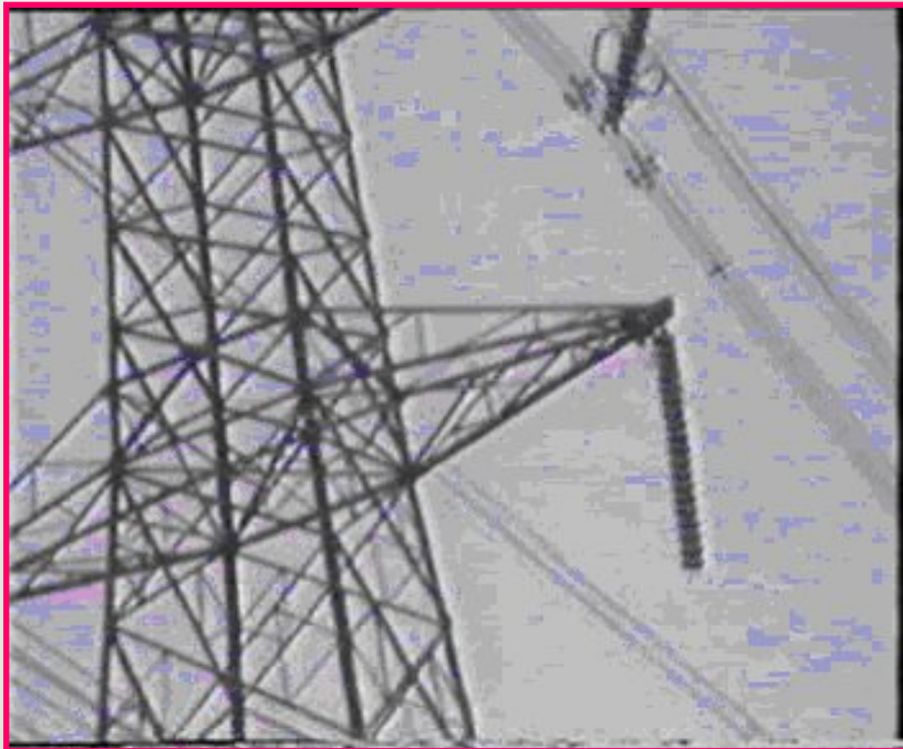
INSULATOR STRING SEPARATED DURING GALLOPING
