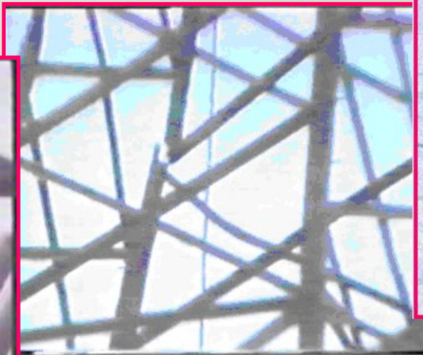
TOWER MAIN LEG BROKEN DURING GALLOPING
