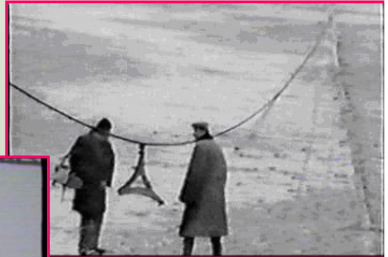
SPACER DAMPER BROKEN DUE TO GALLOPING
