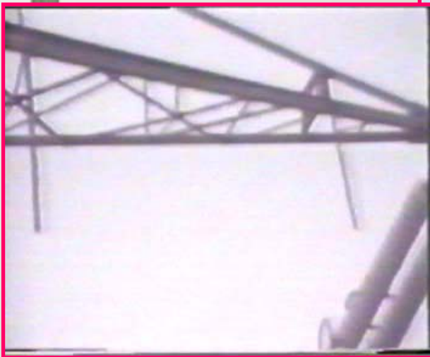
TOWER ARM BRACING MEMBERS BROKEN DUE TO GALLOPING
