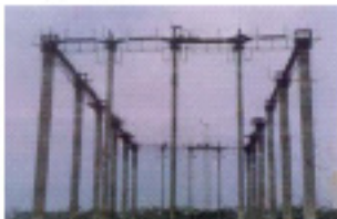
Slipforming of 24 Nos. columns (22 m height) without beam for Bagasse Shed for Balrampur Sugar mill, Gonda UP - First time in the history of Slipforming in India
