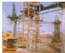
Civil & structural work for Captive power plant at Belrampur Sugar Mills, Gonda
