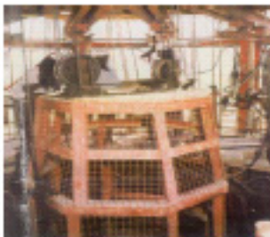
Safety check of Passenger lift before commencing slipforming for 90m taper chimney at OCFL, Orissa
