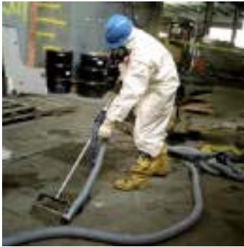
Vacuuming parts of our Taipo's plant
