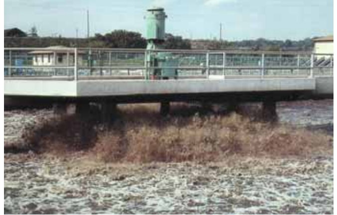
Surface Aerator – Activated Sludge WTP
