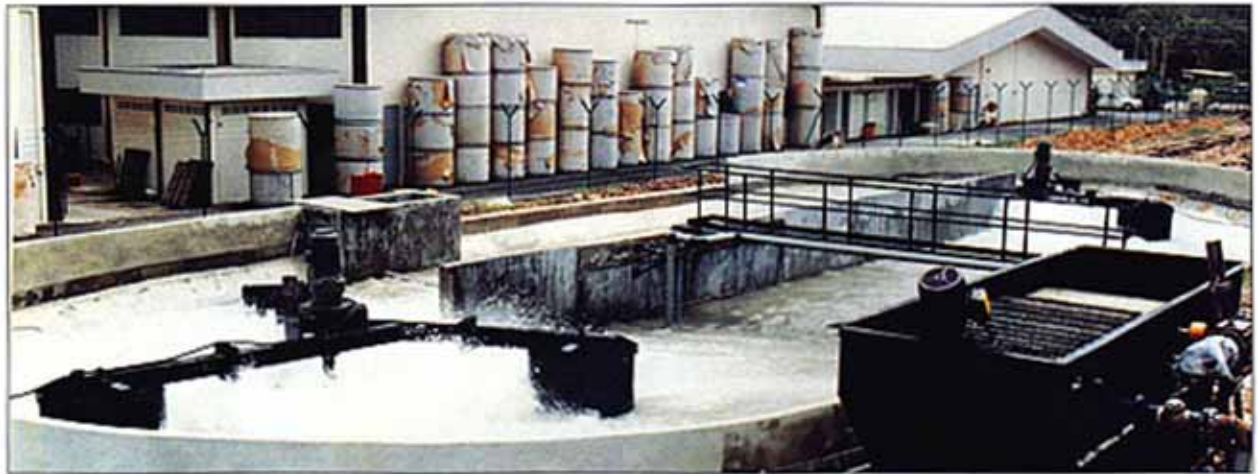
峇株株车害 S & P Coconut 椰粉制造厂 100m 3 /日 氧化沟生活及处理厂 S & P Coconut, Batu Pahat coconut milk processing plant 100m 3 /D Oxidation Ditch WWTP
