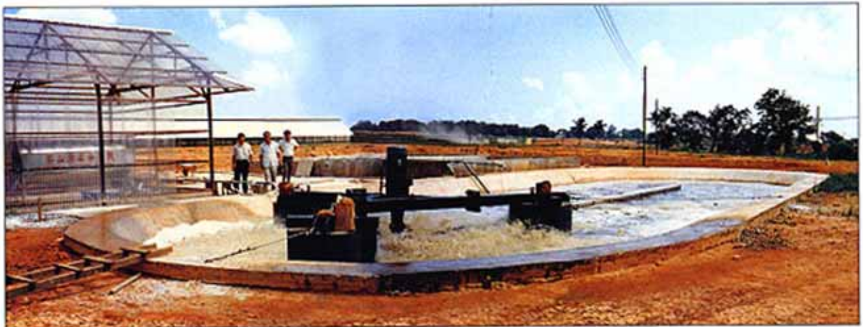
兴隆杨鸭农场 250000鸭只氧化沟污水处理厂 Heng Duck Farm 250,000 Ducks Oxidation Ditch WWTP
