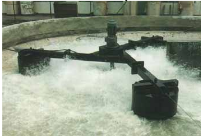
F.O.G WTP – Floating aerator
